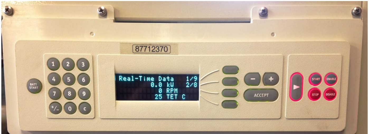
Capstone operator control panel
