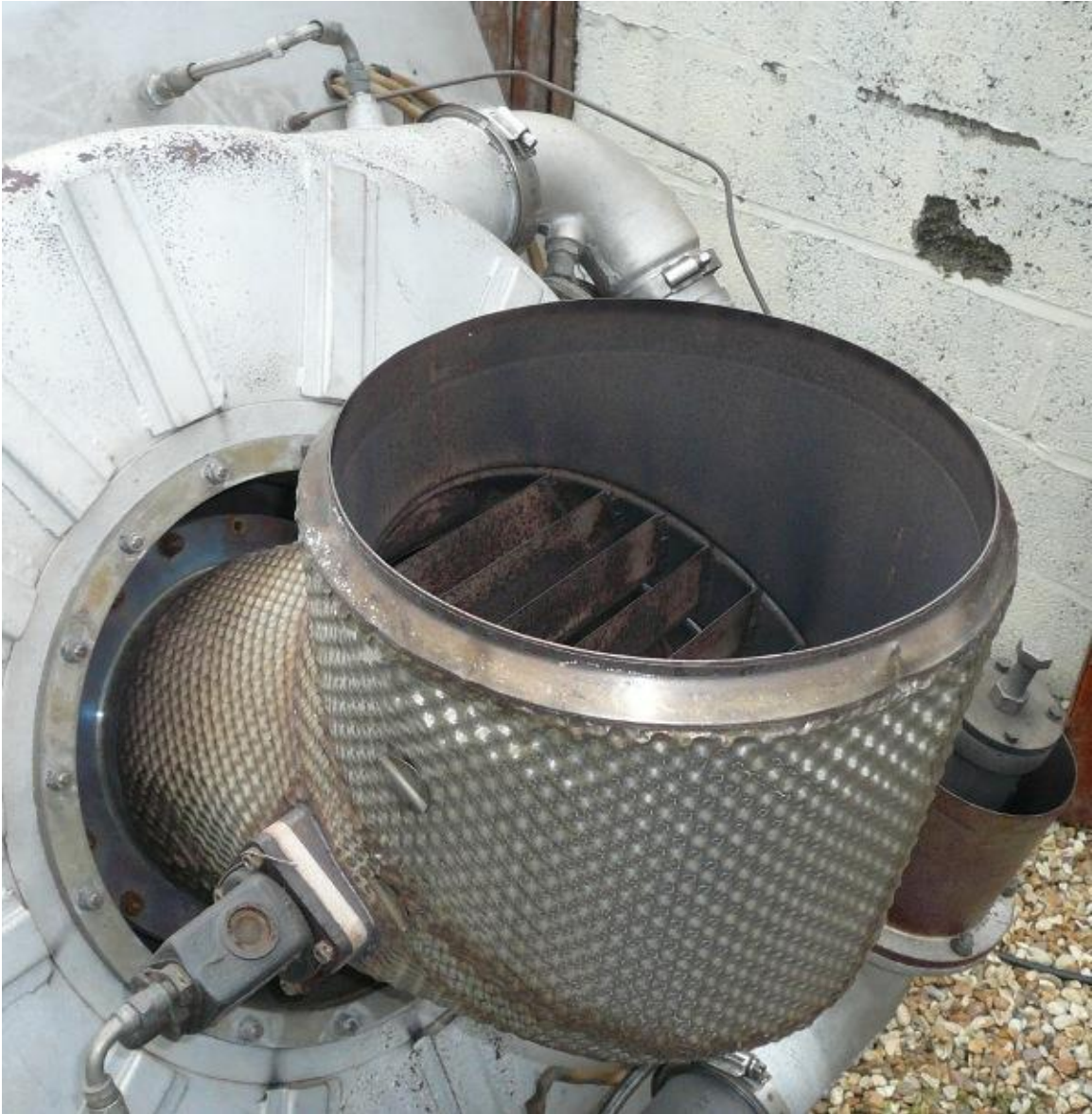
Angled exhaust duct fitted with louver/guides to improve exhaust gas flow
