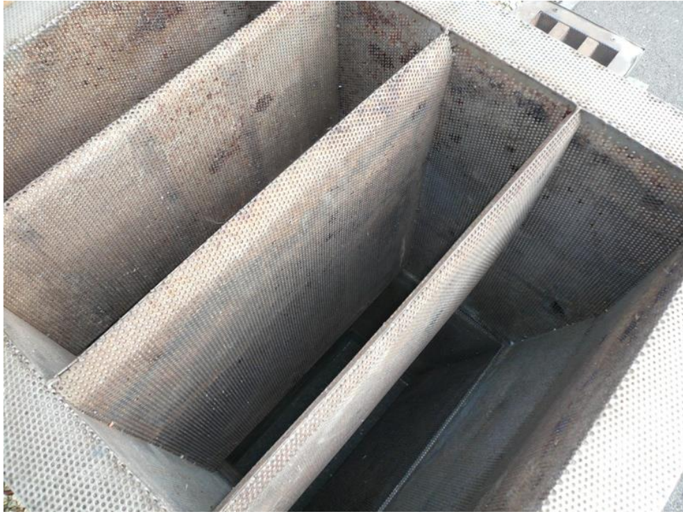
Acoustic splitters in exhaust unit
